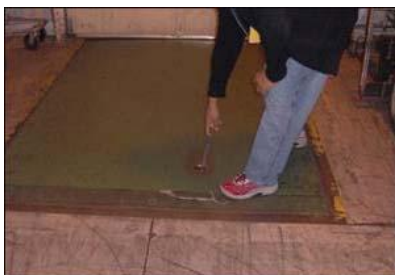
Before - Reaching to the floor to pull a chain that activates the dock leveler
